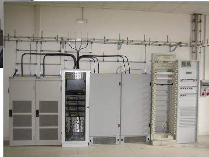
Siemens BTS, Radio Bench, Nortel BTS
